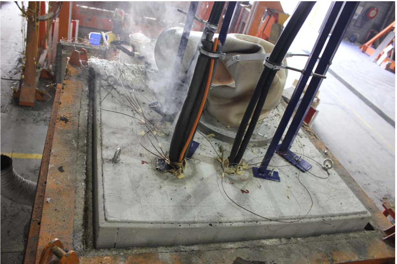
PHOTOGRAPH 7 – PENETRATIONS AFTER 180 MINUTES OF TESTING
